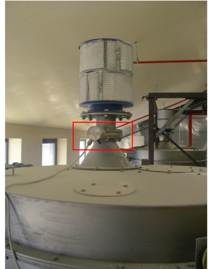
Installed DYNAguard K in cacao powder silo
