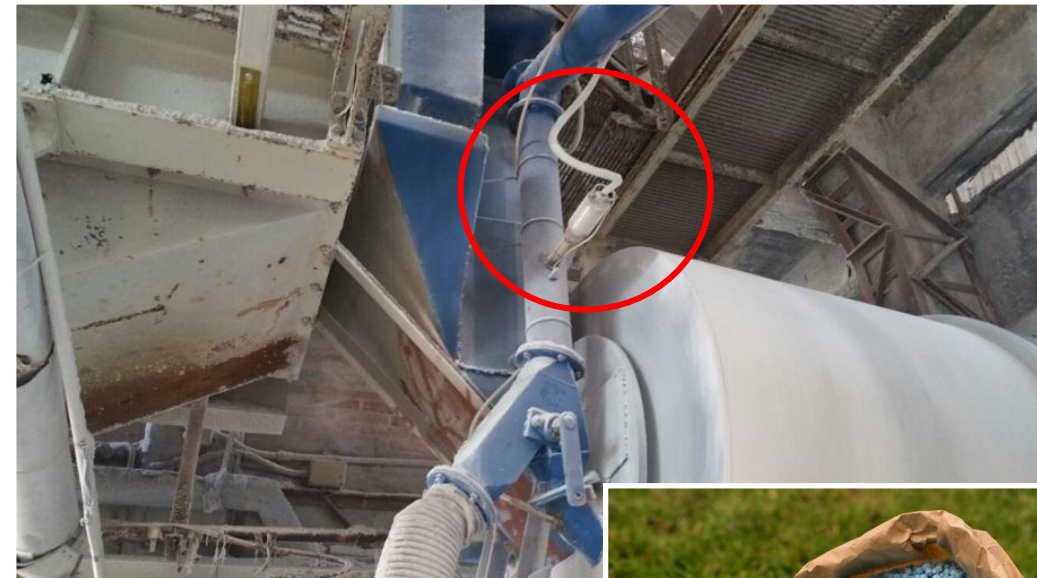
Installed DYNAmflow between auger and granulator.
